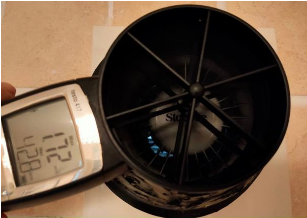
The primary source of vapour comes from the bathroom. Here the extractor fan is manual. The speed was fast. However the extractor fan should be kept on for 30 minutes after showering with the door kept closed.
